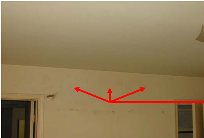
Second bedroom west wall at ceiling opposite shower.
