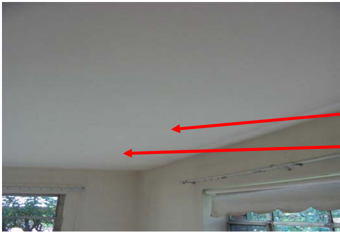
Second bedroom southeast corner ceiling.
